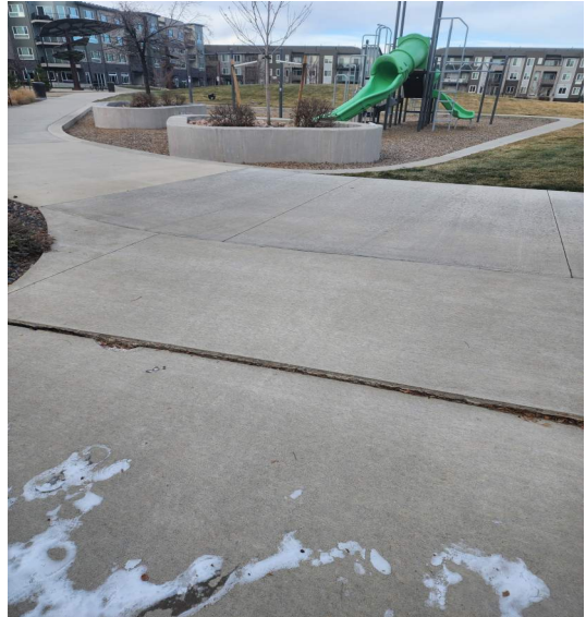
2. Raised concrete at Park Steps.
