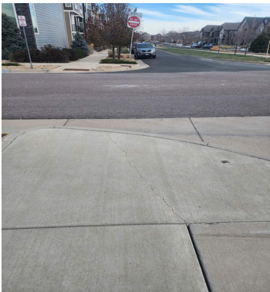
3. Cracked Concrete by ADA Ramp.
