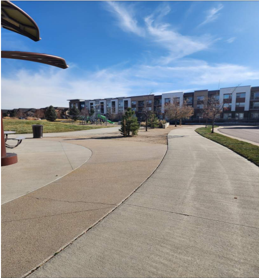
1. Cracked concrete at the Park.
