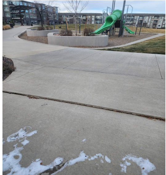
2. Raised concrete at Park Steps.
