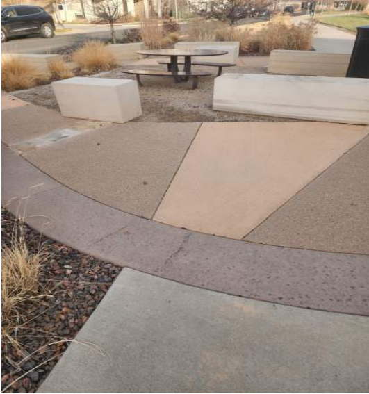
6. Cracked concrete at center sitting area at East Dry Creek PL.
