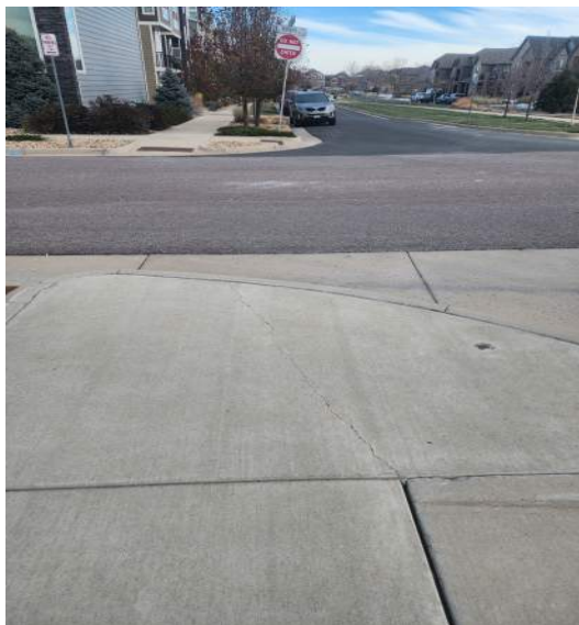
3. Cracked Concrete by ADA Ramp.
