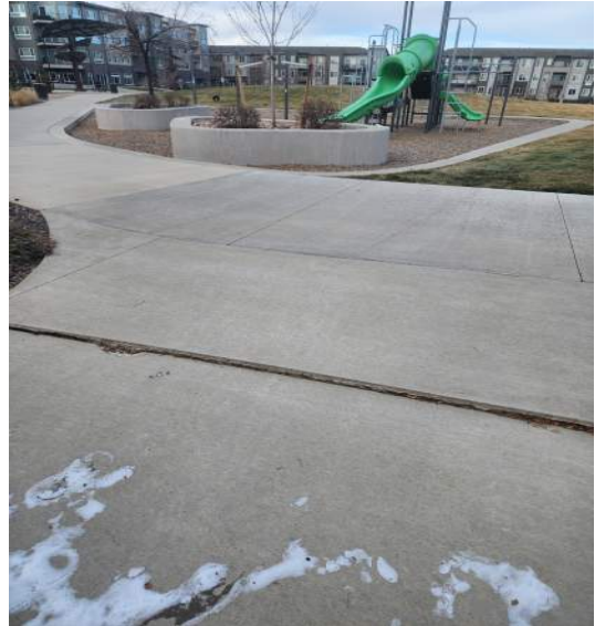
2. Raised concrete at Park Steps.
