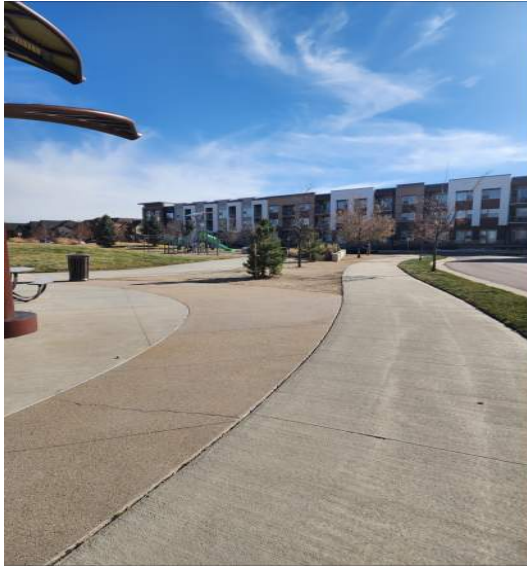
1. Cracked concrete at the Park.
